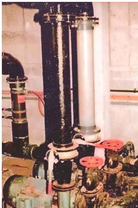
Figure 1.3 An example of metal corrosion and replacement of a length of corroded metal pipe with a plastic alternative
